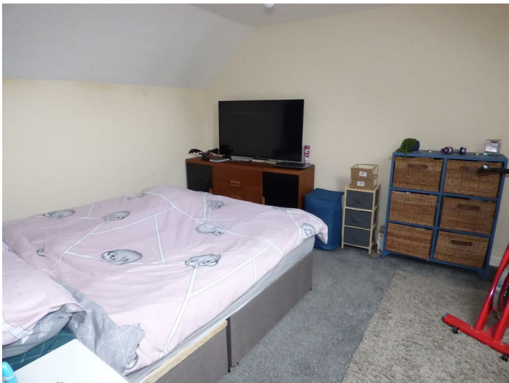
Radiator and Velux window
